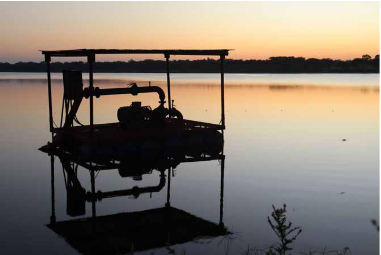
Water pump at the Kasisi Dam
